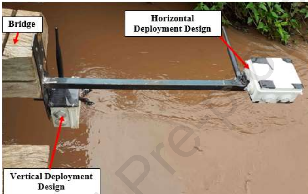
Figure 14: Deployed Sensor Node (Horizontal Deployment Design – 2)
