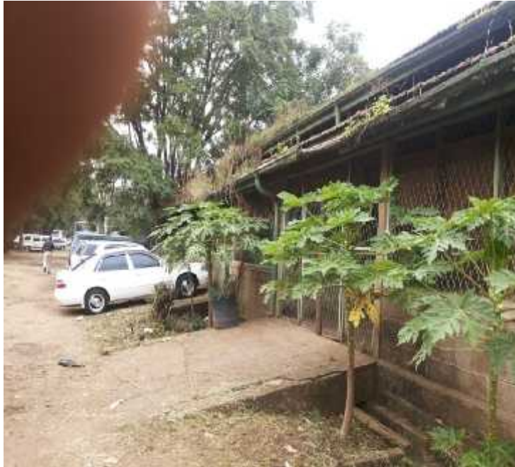
Gutters without provision for maintenance
