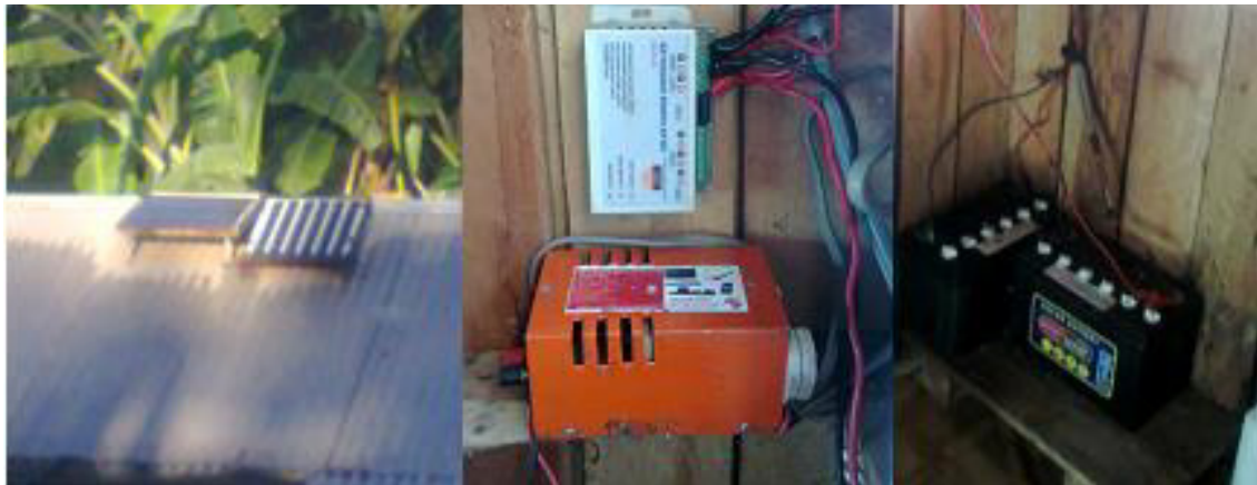
Fig. 8. Typical Solar Home System (a) Panels; (b) Charger controller and Inverter; (c) Batteries
